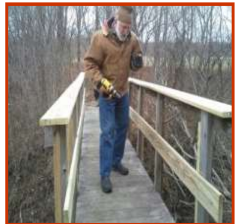
Dan Smith does a final check of bridge repairs at the Galway Preserve
